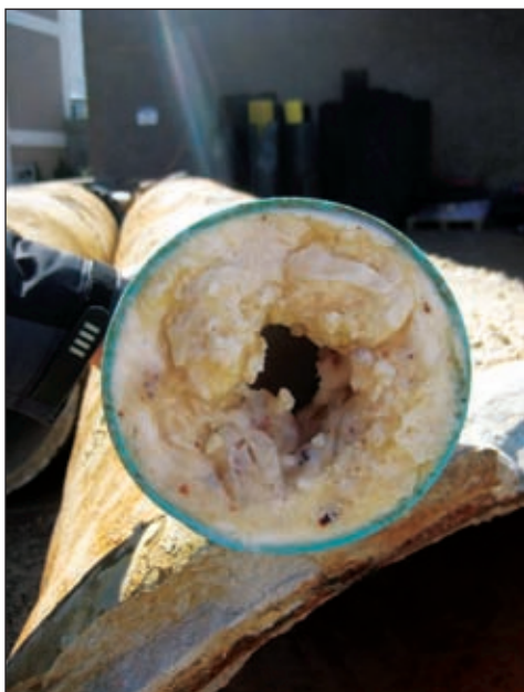
Fats, oils and greases of all types can clog pipes and lead to backups.
