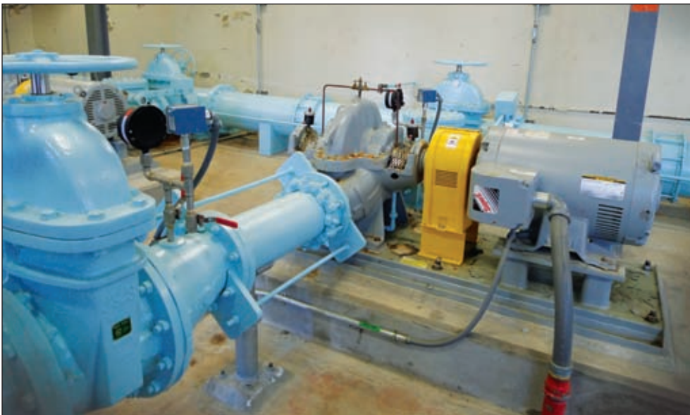
This is one of several pumps at the Lee Pumping Station, which was upgraded in 2011.
