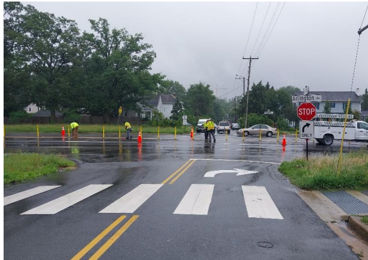
Installation of tactical median closure at the intersection of Route 50 and Highland St
