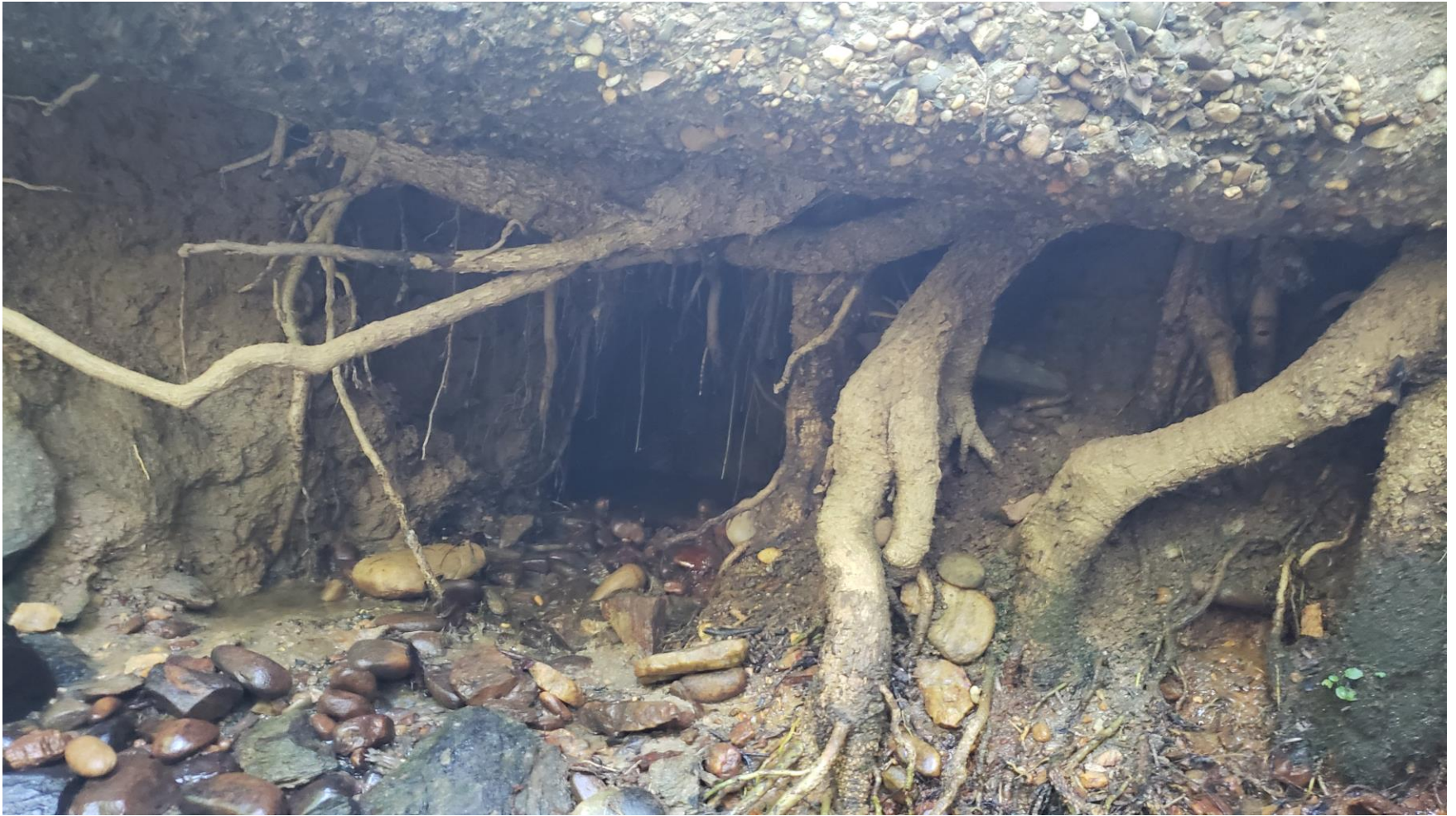
August 2025: Water drips through a hole in the concrete pad, continuing to undermine the structure.
