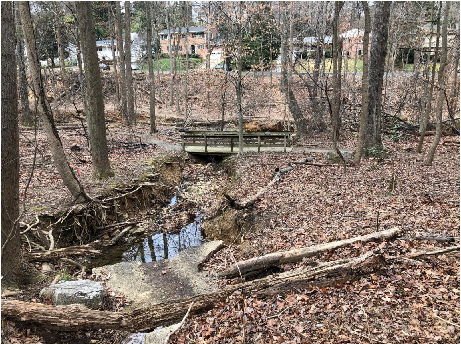
January 2020, View from upslope of the outfall toward Gulf Branch stream and 36 th Rd N
