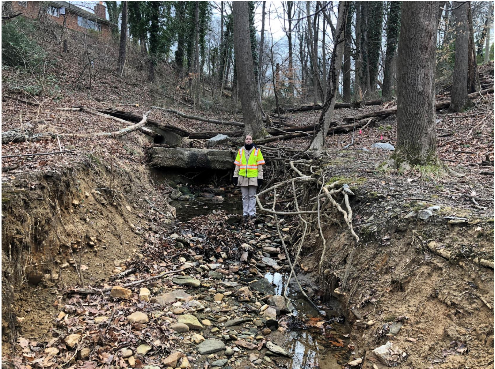
January 2020 Erosion undermining endwall and concrete pad
