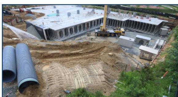
Cardinal Elementary Stormwater Vault
