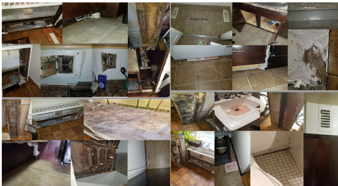
Figure 1 – Pictures of conditions in multiple units at Serrano Apartments from NAACP Letter to Arlington County dated April 30, 2021
