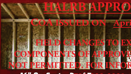
16" On-Center Roof Trusses
