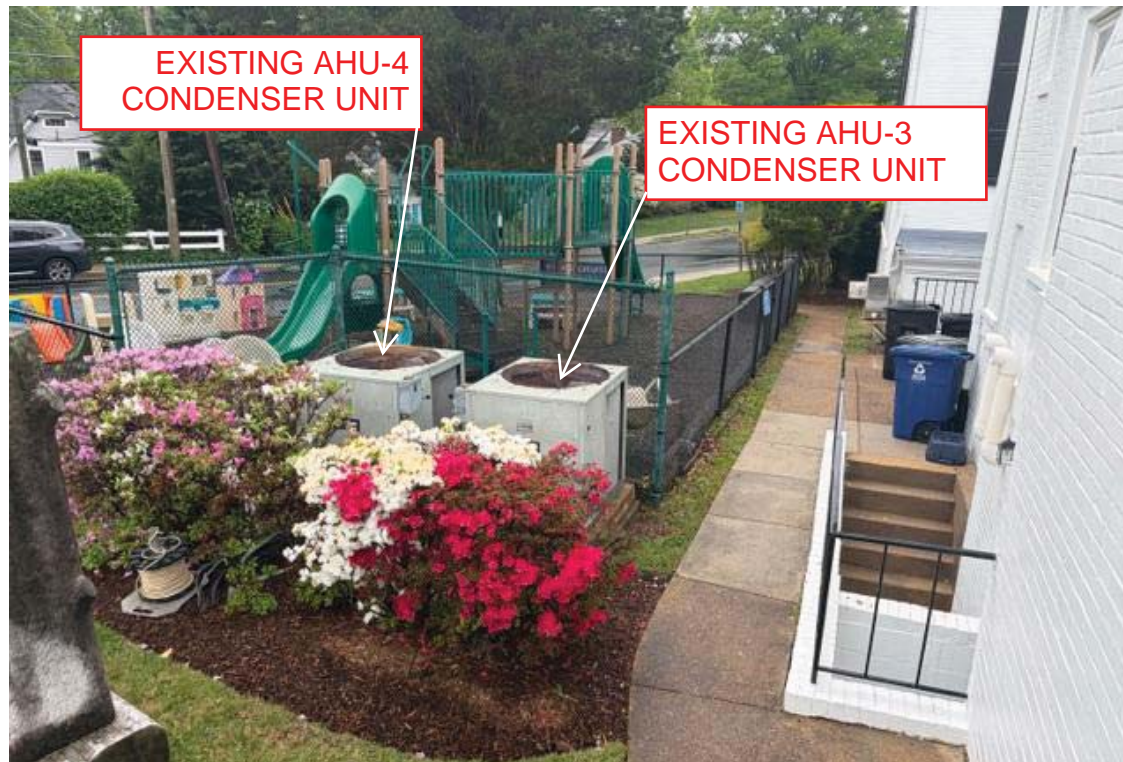
VIEW OF CURRENT MIDDLE AND LOWER LEVEL CONDENSER UNITS
