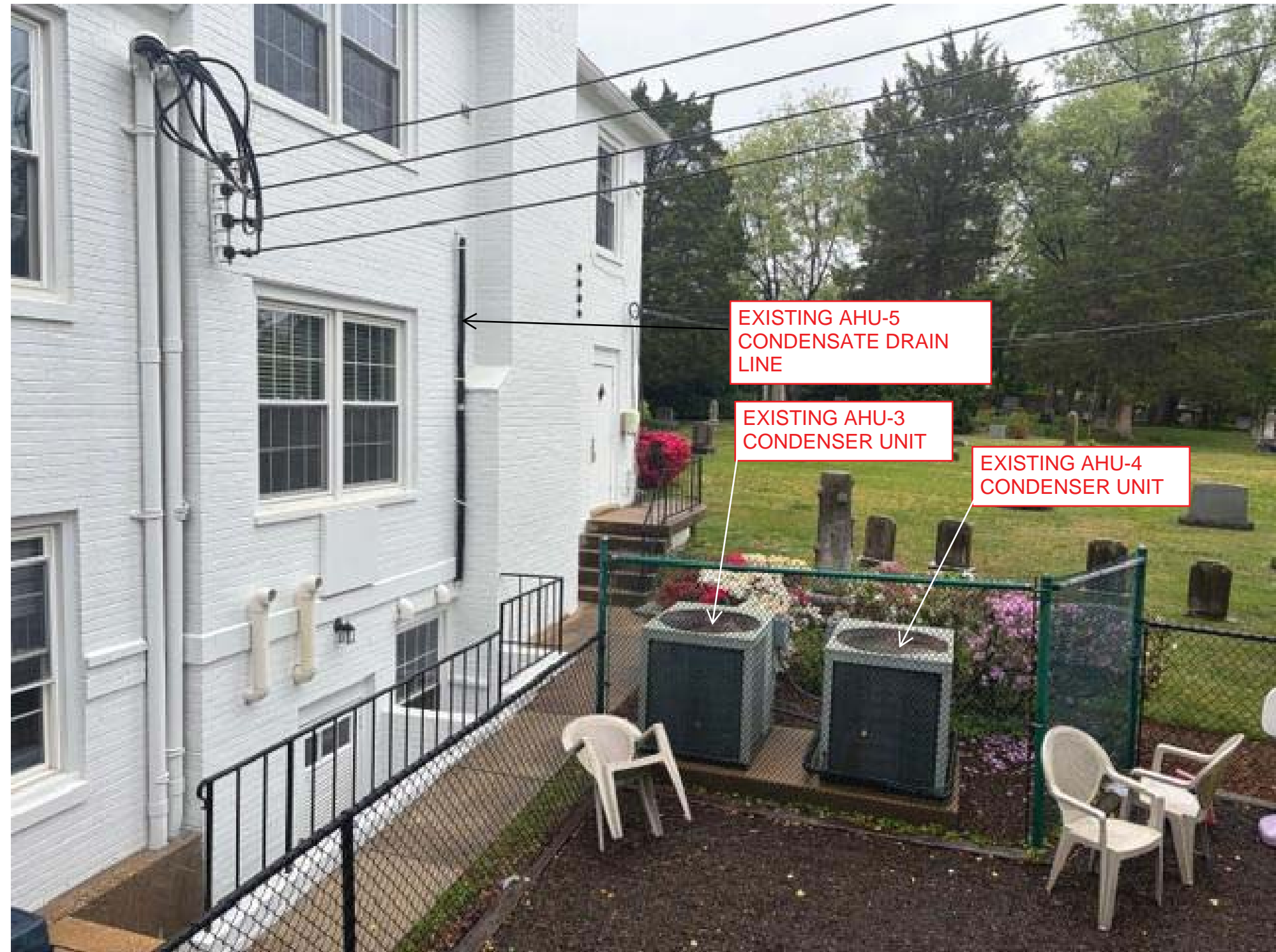
VIEW OF CURRENT MIDDLE AND LOWER LEVEL CONDENSER UNITS FROM ATOP THE PRESCHOOL PLAYGROUND EQUIPMENT
