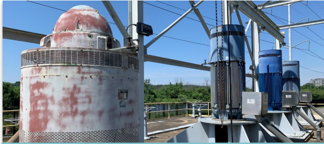
Activated Sludge Effluent Pump Station #1 (ASE1)
