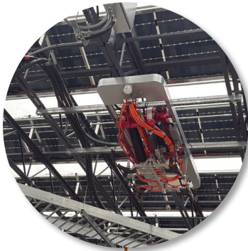
Bus Charging Equipment at AOMF
