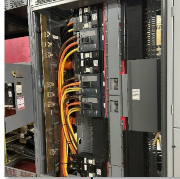
Courts/Police Electrical Re-Commissioning
