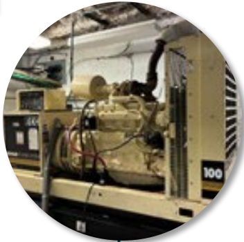
Generator Replacement Program - CSI
