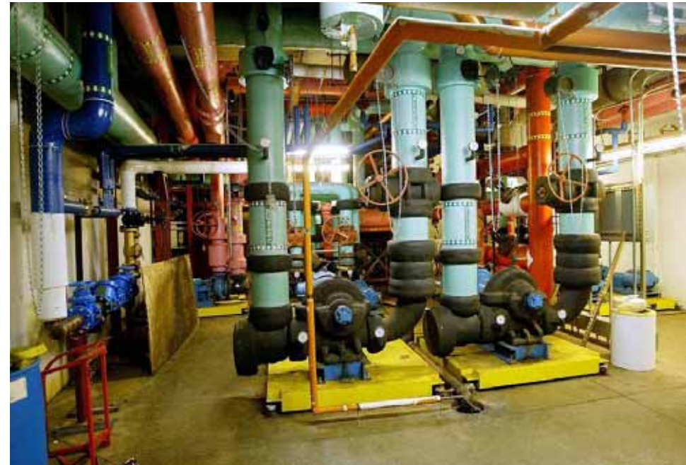
Mechanical Control Systems Gaylord Entertainment Center Nashville, Tenn. Architect: HOK Sport+Venue+Event
